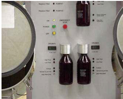
Close up of bubbler and controls
